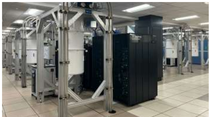
Figure 317: IBM's quantum data center in Poughkeepsie, New York State. Source: IBM.
