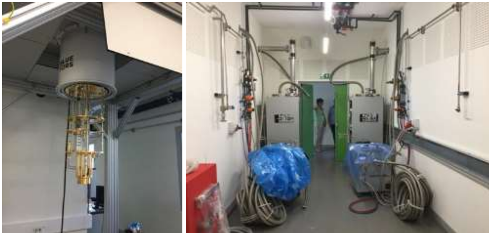
Figure 493: Bluefors installation at CEA IRIG in Grenoble. Photos: Olivier Ezratty. 2019.
