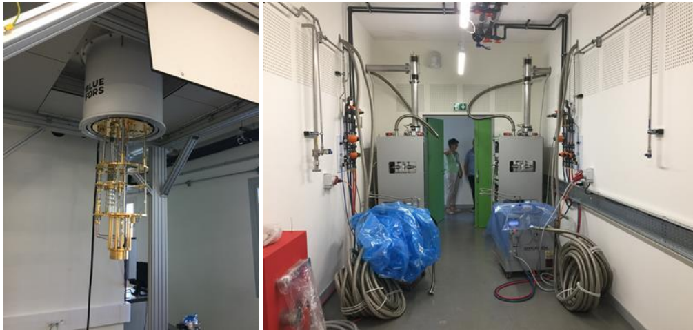
Figure 465: Bluefors installation at CEA IRIG in Grenoble. Photos: Olivier Ezratty.
