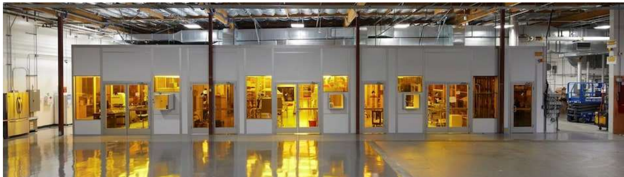
Figure 326: Rigetti's superconducting cleanroom fab line in Fremont, California. Source: Rigetti.
