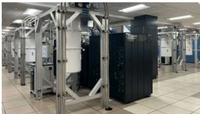
Figure 305: IBM's quantum data center in Poughkeepsie, New York State. Source: IBM.
