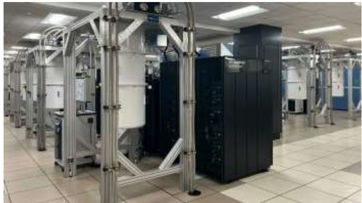
Figure 305: IBM's quantum data center in Poughkeepsie, New York State. Source: IBM.
