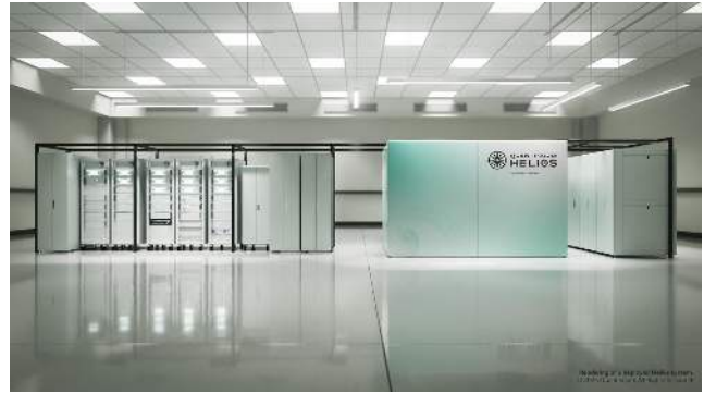
Figure 213: Quantinuum Helios installation shows on the right the experiment location and on the left all the racks with laser and control electronics. The system cryogenics is fed a helium liquefier. It cools the ions chamber at about 15 K. The total system power is of about 34 kW. Source: Quantinuum, November 2025.
