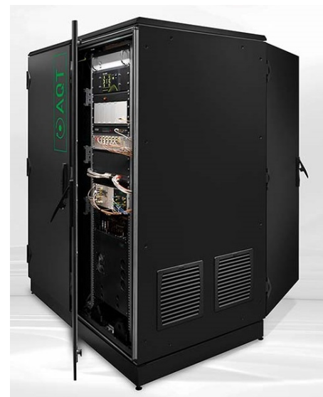
Figure 229: AQT 2-rack system. It consumes about 2 kW.
